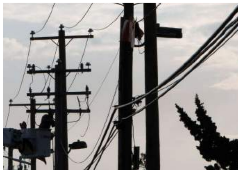
Restoration of electricity, Long Island, New York (United States). Elec nor Hawkeye
