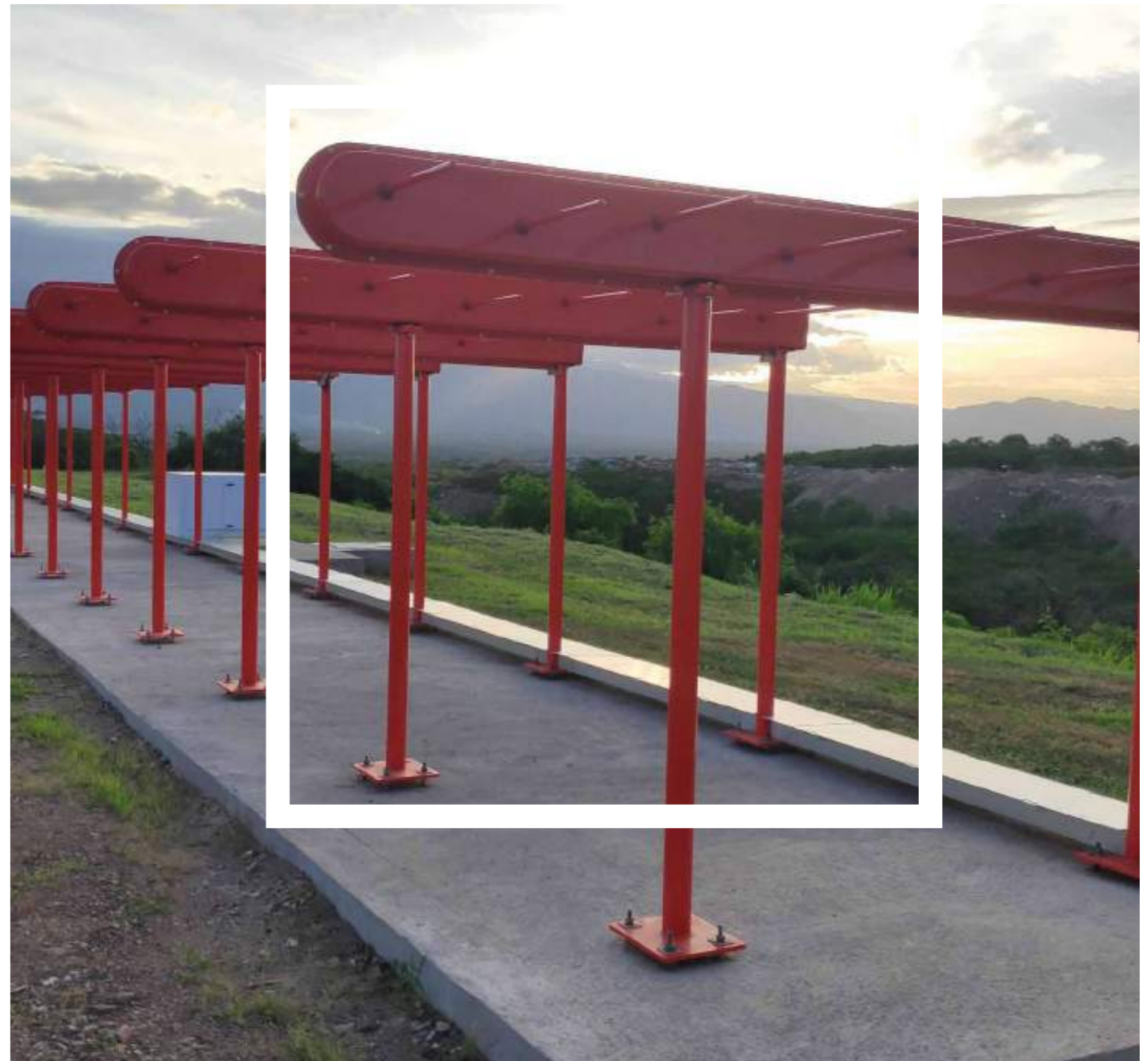
ADS-B system at the Palmerola Airport (Honduras)
